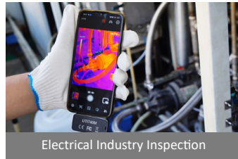
Distribution Cabinet Inspection
